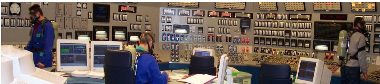
Figure 16: Operators Using Breathing Apparatus in Case of Toxic Atmosphere in Main Control Room (Simulator)
