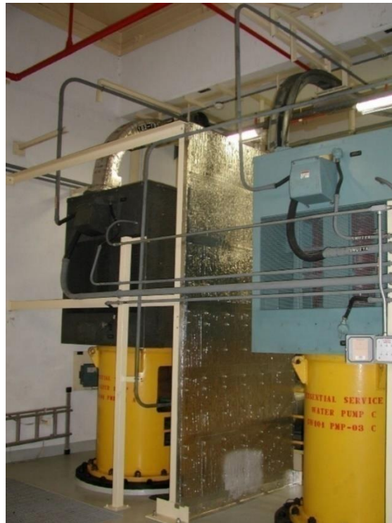
Figure 23: Fire Barrier between Service Water Pumps
