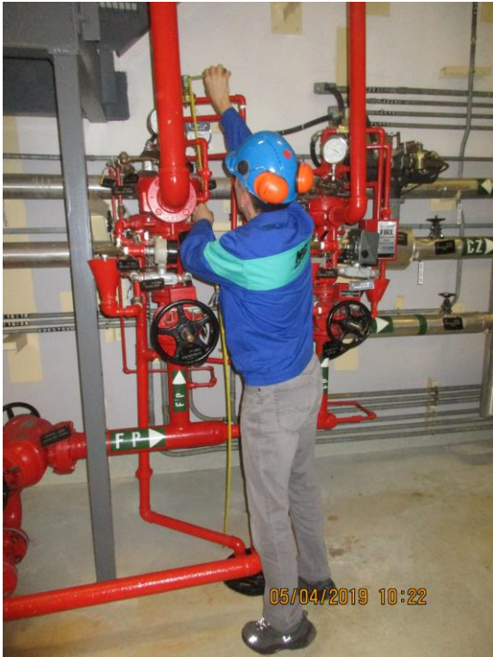
Figure 46: Testing of MCR Charcoal Filter Fire Extinguishing System
