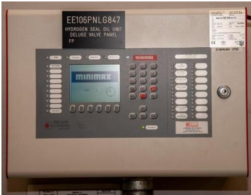
Figure 35: New Control Panel for Fixed Fire Extinguishing System
