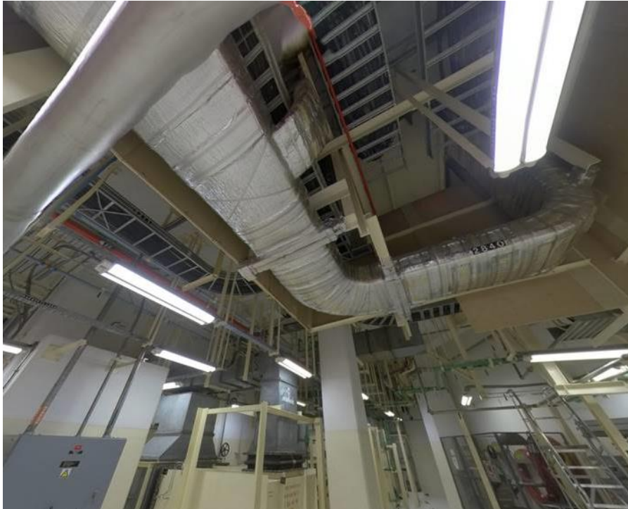
Figure 22: Wrapped Cables in Auxiliary Building
