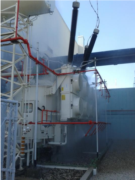
Figure 45: Operational Testing of Main Transformer Fire Extinguishing System
