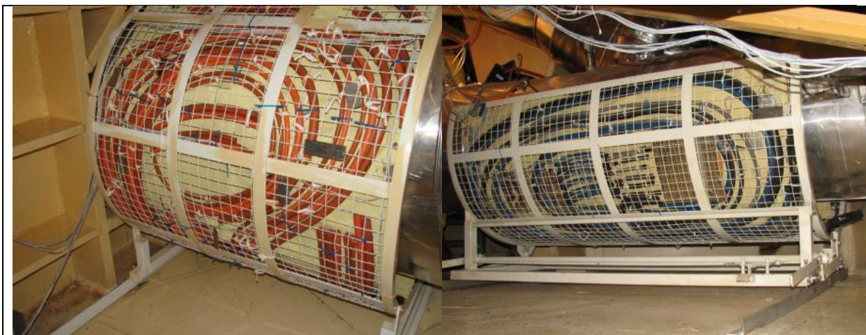
Fig. 3.3: Deposits with surveillance cables
